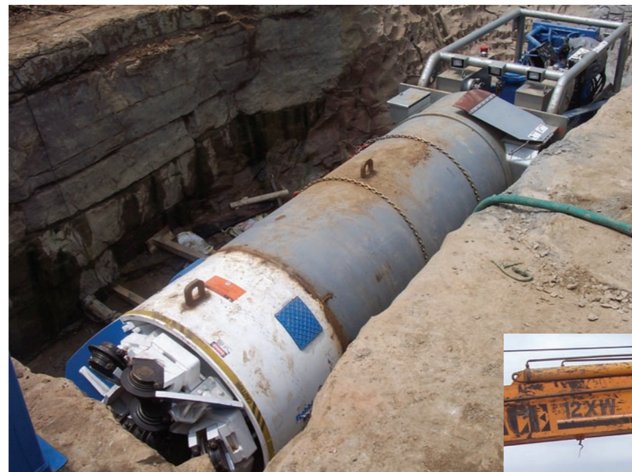
Left: The 1.5 metres Robbins SBU-A excavated two 50 metre crossings after three unsuccessful attempts with other methods.
